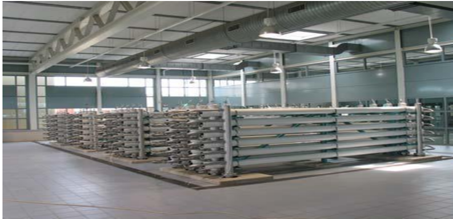
Figure 4: UF Plant at Heemskerk, the Netherlands
