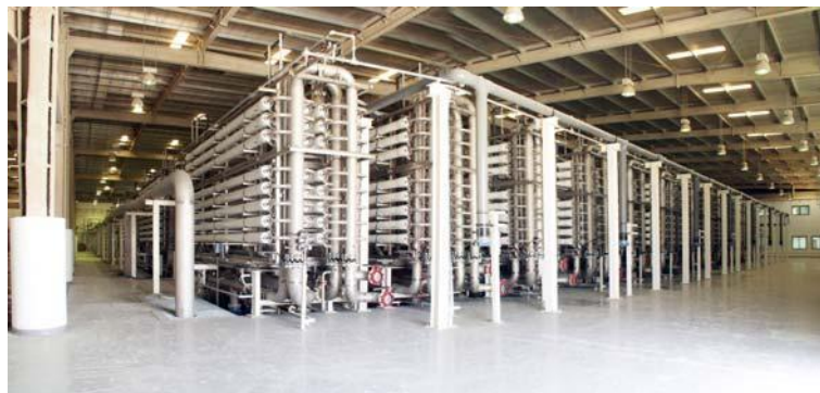
Figure 3: UF Plant at Sulaibiya, Kuwait
