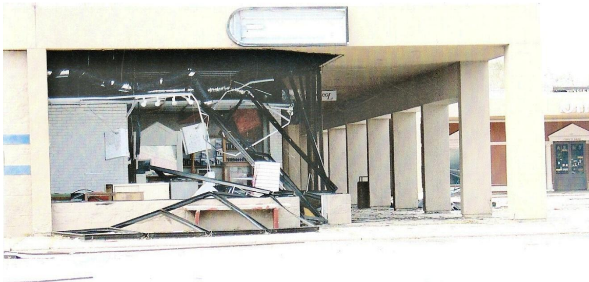
Figure 1: Lookin Good Hair Salon Hurricane Rita Damage
